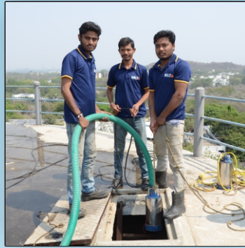
For Dewatering Imported Vacuum Pump or high discharge Pump Is used as per site conditions
