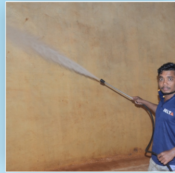
High pressure jet with variable Pressure is used for cleaning, corners, walls & base of the tank
