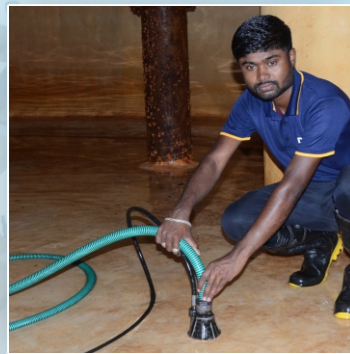
Vacuum Sludge Pump is used to dispose the dirty water & sludge from the tank
